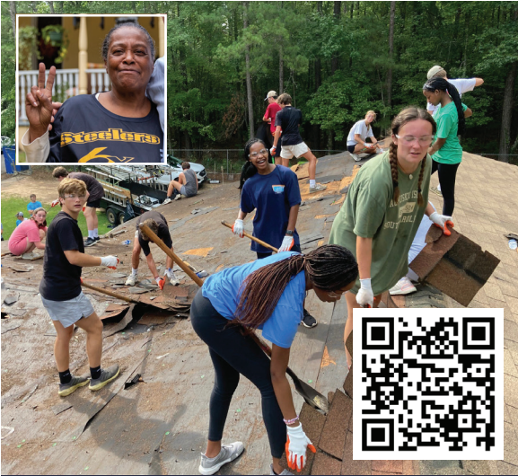
Albertha Taylor's home was repaired thanks to United Way, Home Works, and volunteers like these.
